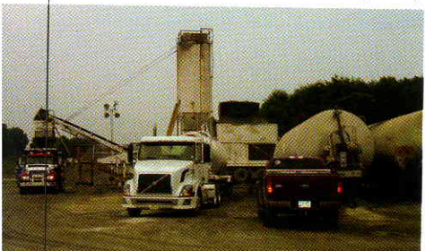
The RCC material is being manufactured on-site in a continuous pug-mill operation. This unit, an Aran ASR280B, produces RCC at rates of up to 500 tons per hour.
